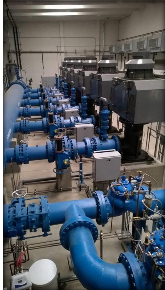
Image 13. High Service Pump Station
