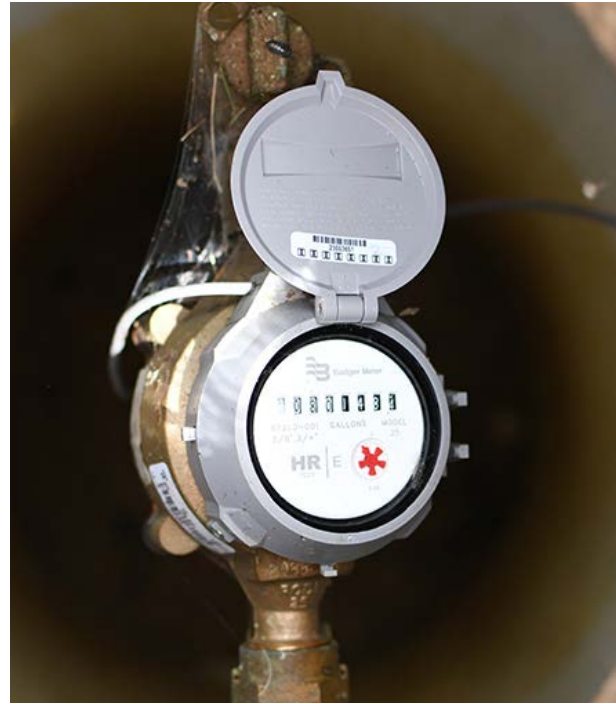
Image 18. AMI Water Meter
